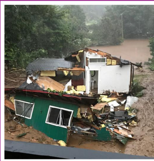
Almost 6,800 people and 95 critical facilities exposed to 1% annual chance flood 5
