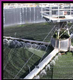
Water and power systems
